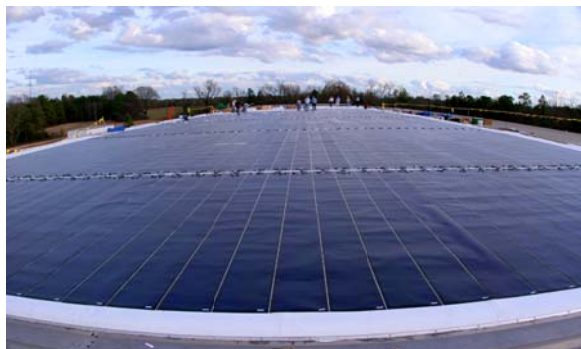
Figure 1, HCO 107.7 KW BIPV Solar System in Benson, NC.
